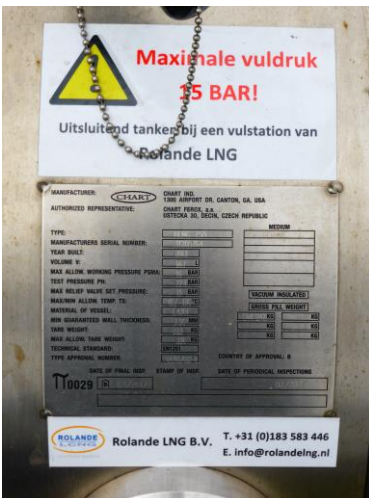
Specifications of the LNG tank and contact details of the operator are on the fuel tank.
